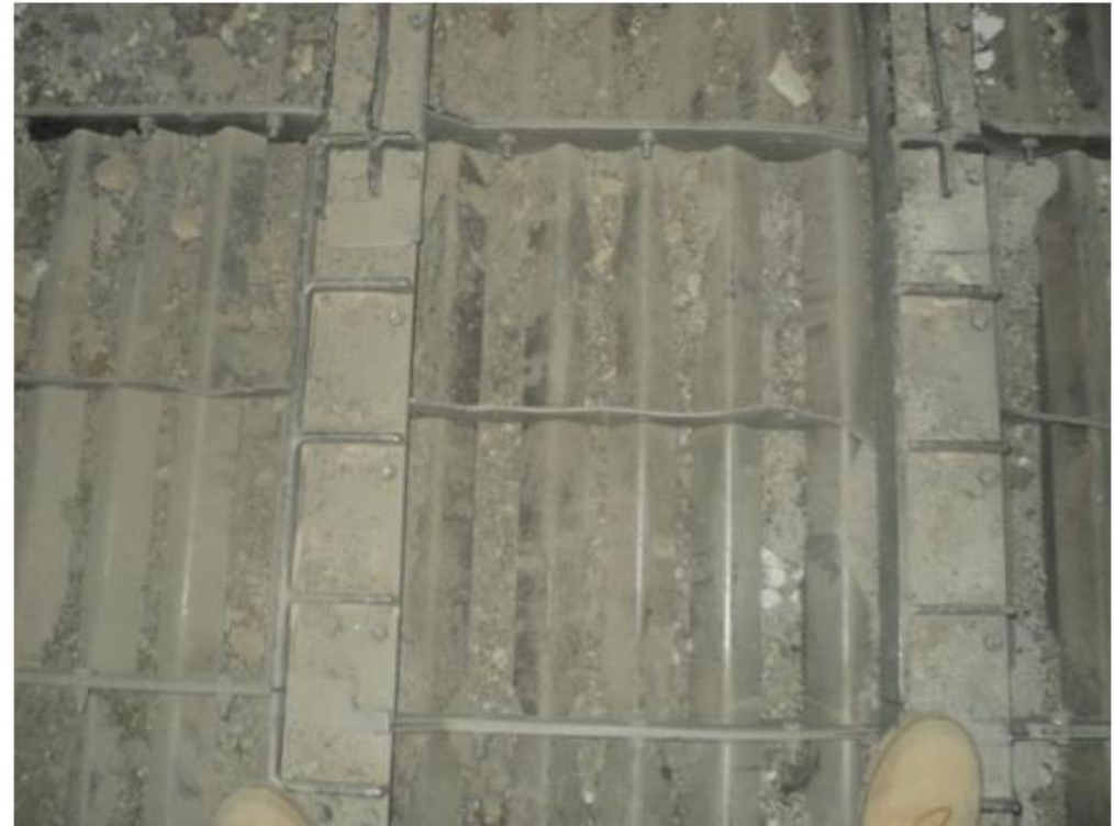
Aeration Cassettes after 7 years of operation In 2014.
