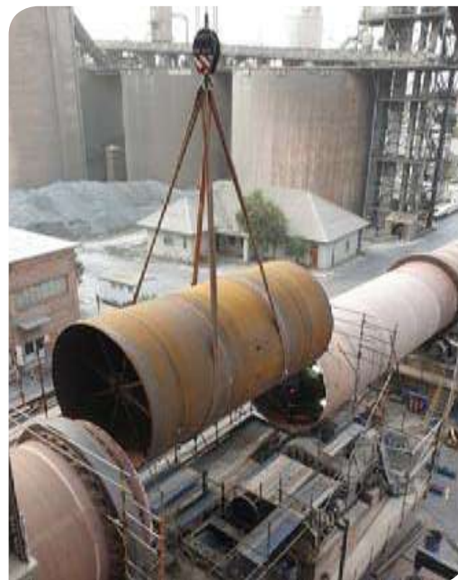
Above left: Daylight between the damaged and undamaged kiln sections after cutting.
