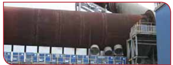
Above: Section of the kiln at the Martinsburg cement plant in West Virginia, USA.
