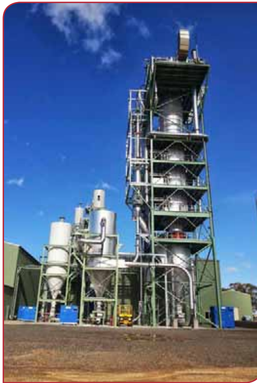
Left - Figure 2: Calix's Bacchus Marsh plant in Australia has used a Direct Separation Reactor (DSR) to produce niche 'extremely caustic MgO' since 2012, while trapping the plant's process CO 2 emissions.
