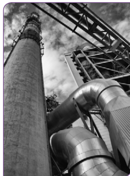
Above - Honourable Mention: Stanislaw Dunin-Borkowski, Elements of the pre-heater tower at cement plant in Ozarow, Grupa Ozarow SA, Poland
