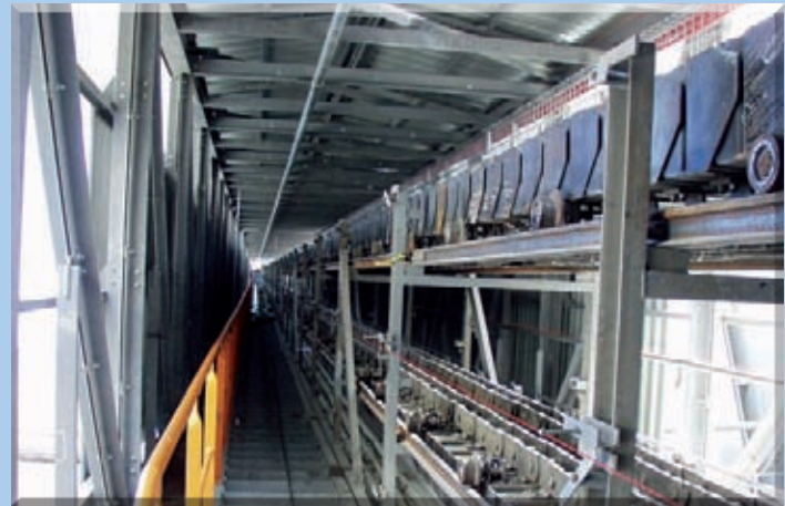
Clinker pan conveyor
