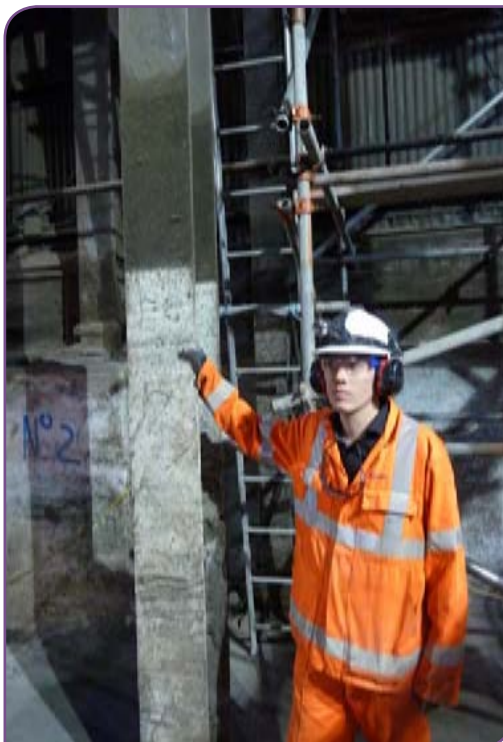
Left: Damian Marsden, the plant’s Engineering Development Manager, stands next to a beam inside the plant. The high water mark is clearly visible, some 80-90cm above his head.
