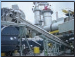
Chain Conveyors Conveying up to 1,000 t/h
