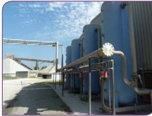
Left: Several separate compressed air stations were centralised into a single facility as part of the renovation work.
