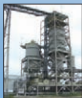
Silo Dischargers Discharging up to 1,000 t/h
