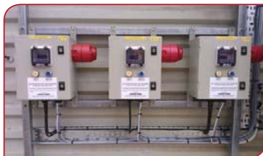
Left: Bespoke alarm panel with GLT and automatic shut off.
