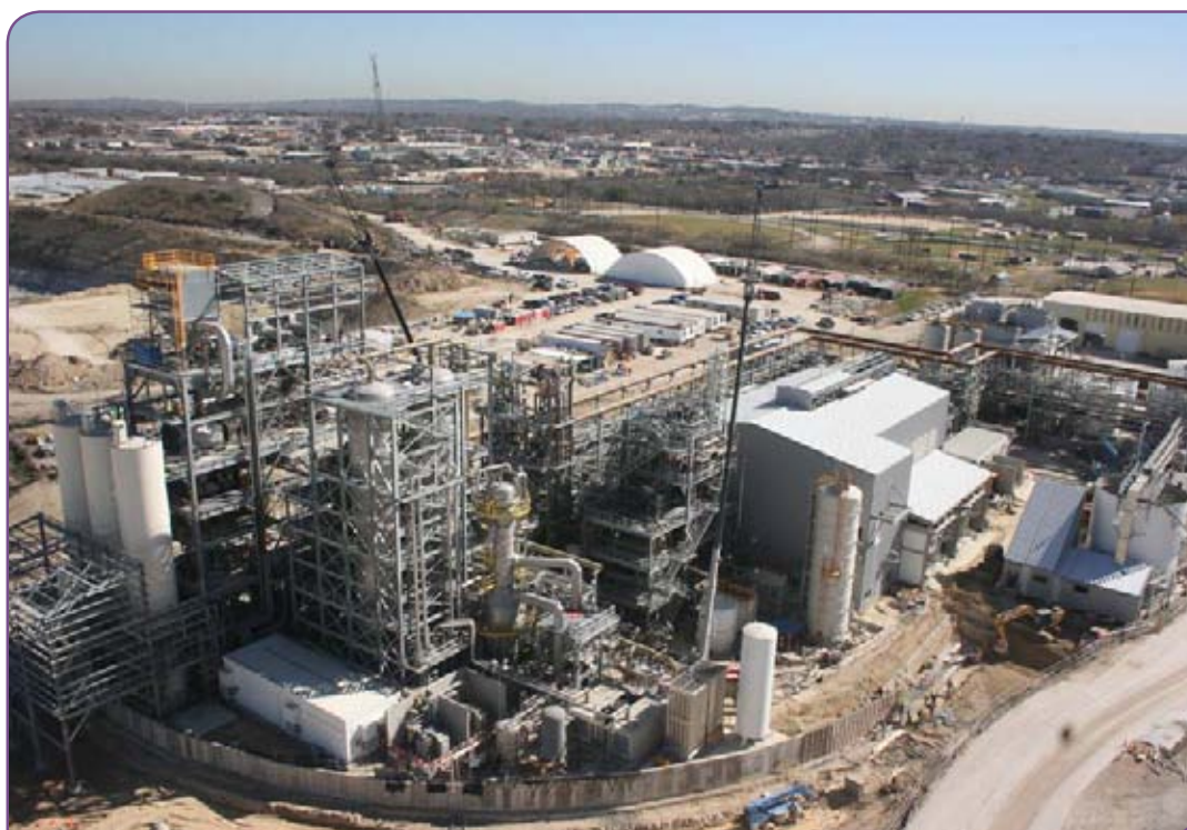
Left: Construction of the Capitol SkyMine, as seen from the adjacent Capitol Cement plant in early 2015.
