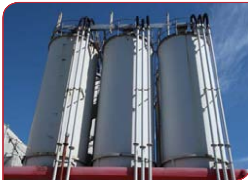
Left: Three of Sika's nine cement and sand silos at its UK headquarters in Welwyn Garden City, Hertfordshire. The nine silos have recently been fitted with SPS Silo Protection Systems from Hycontrol.
