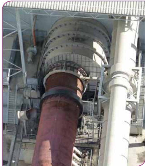
Above: The Akmenes Cement plant was visited by Global Cement in 2015.
