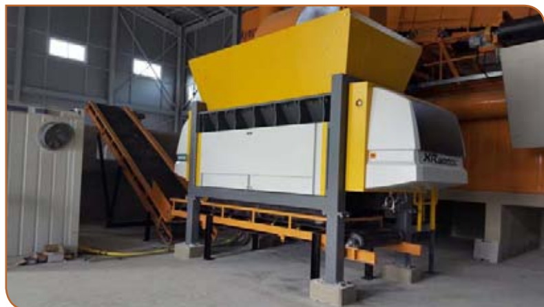
The UNTHA XR3000C shredder installed by Zion in Wonju, South Korea.
