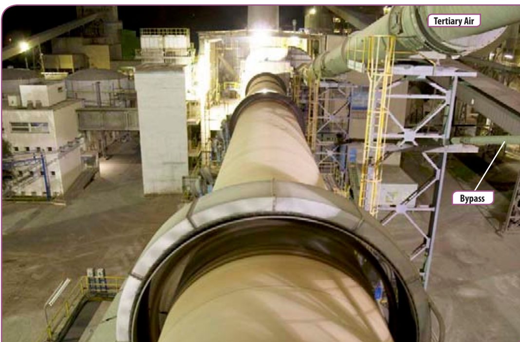
Left: View over the kiln at night with tertiary air duct and bypass.
