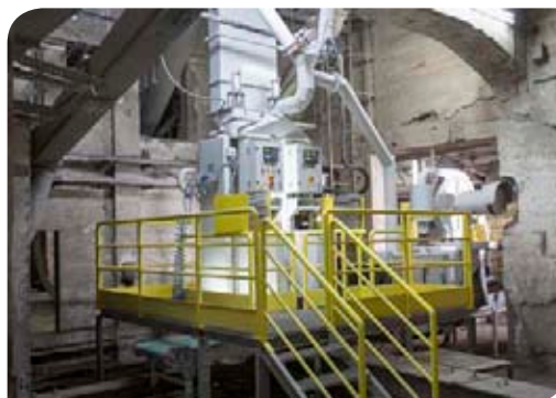
Left: The cement industry normally uses turbine filling machines. However, Calucem opted for a BEUMER fillpac air filling machine, because its cement compositions can vary greatly and are often finer than that of traditional cement.
