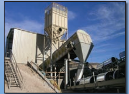
Truck Unloading Stations Receiving up to 1,200 t/h
