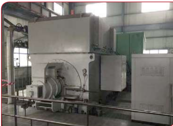
Below - Figure 5: View of the generator.
