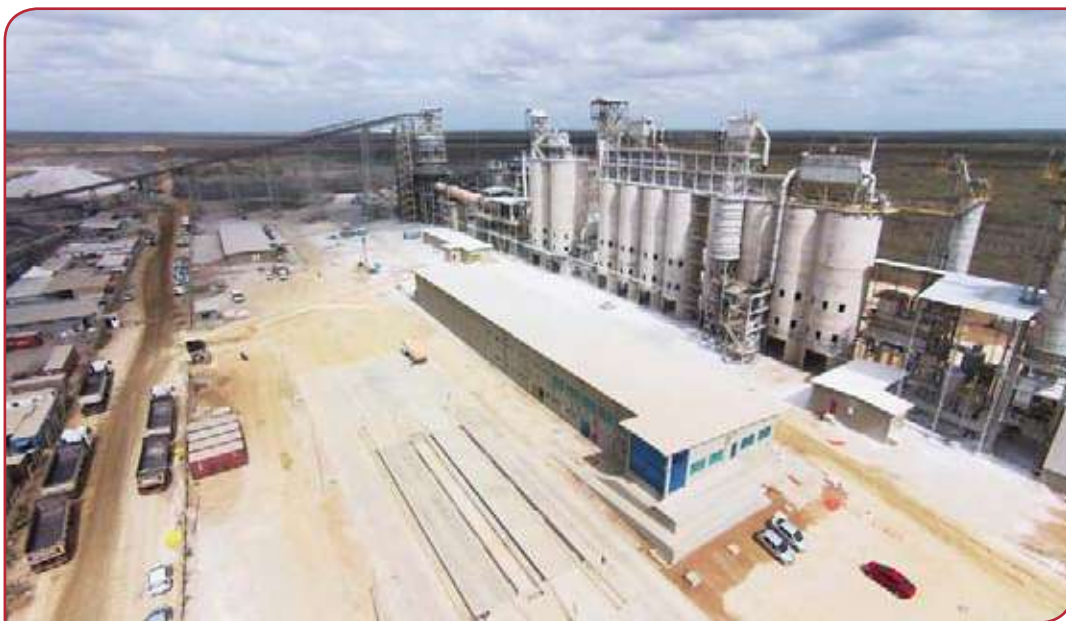
Left - Figure 2: Overview of the lime plant during the commissioning phase
