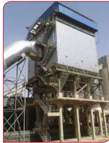
Left - Figure 3: Filter bag installation for the clinker cooler at Southern Province Cement.
