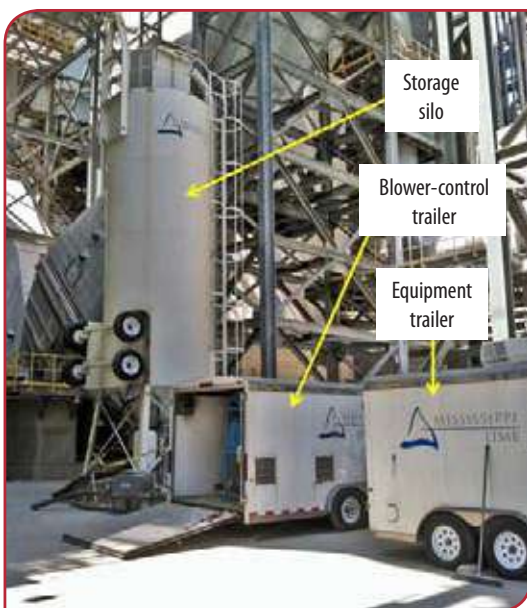
Below - Figure 1: A temporary DSI injection system.
