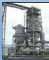
Silo Dischargers Discharging up to 1,000 t/h
