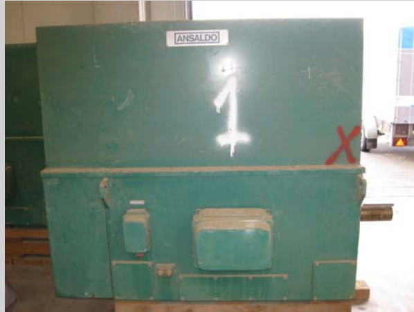
Picture: 5 main drive motor
